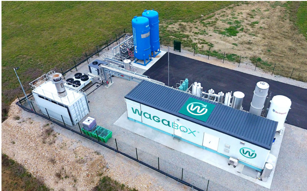
Fig. 34: The WAGABOX® unit installed on the Suez site in Les Ventes-de-Bourse
