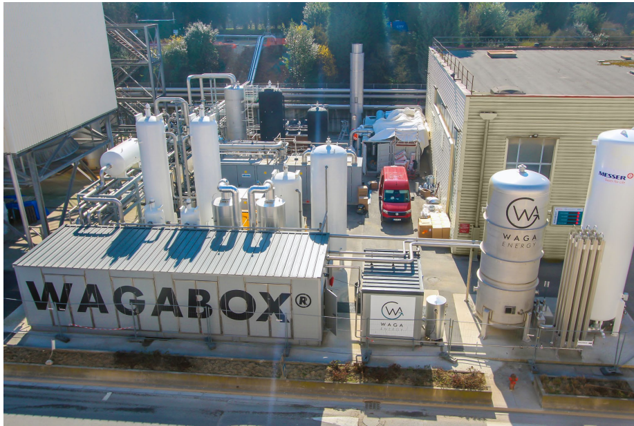
Biomethane production unit installed at the industrial ecology hub operated by Veolia in Claye-Souilly.
